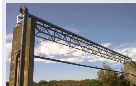
ABOVE Macassar Water Main Link, Macassar, Western Cape (2009): The project entails the construction of a 1.9 km length of 250 mm diameter water main link in Macassar, Western Cape. The route consists of the crossing of a river, an environmental sensitive area and an existing township. CSM Civil and Structural Engineering Divisions were involved in the design of the water main and water crossing structure, and CSM Construction Monitoring Division was involved in contract administration and supervision of the construction
